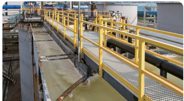
FRP Channel Handrail
