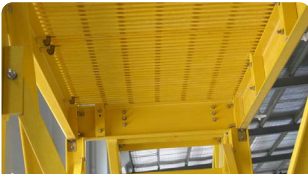
FRP Channel Ladders Supports
