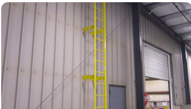
FRP fixed ladder for roof access.
