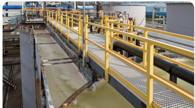
FRP Channel Handrail
