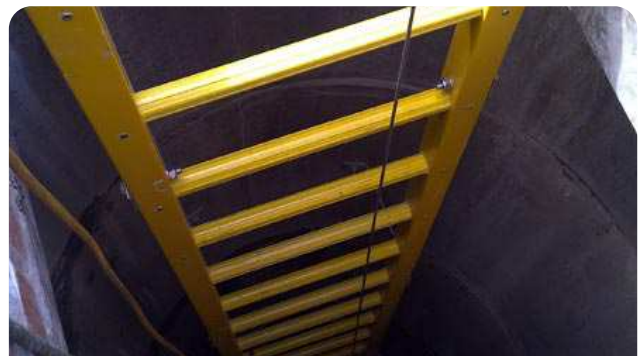
FRP fixed ladder for deep well access
