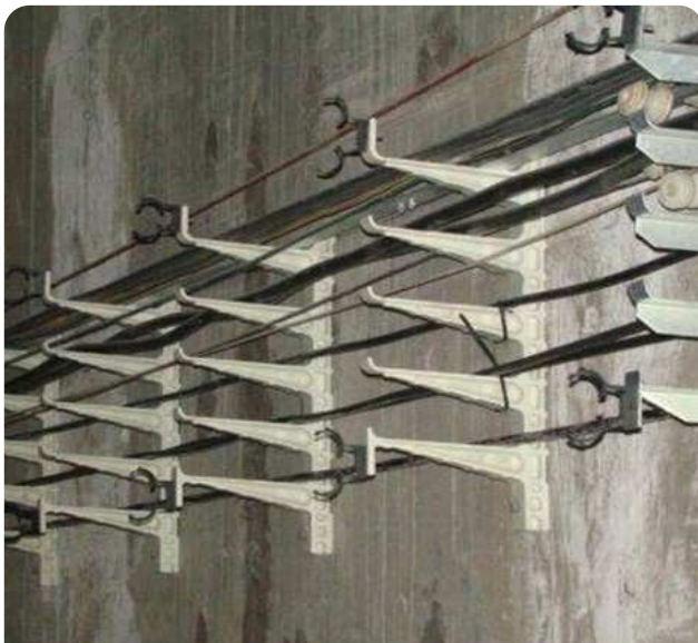
FRP cable bracket in cable tunnels
