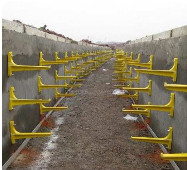
FRP cable bracket in cable trenches
