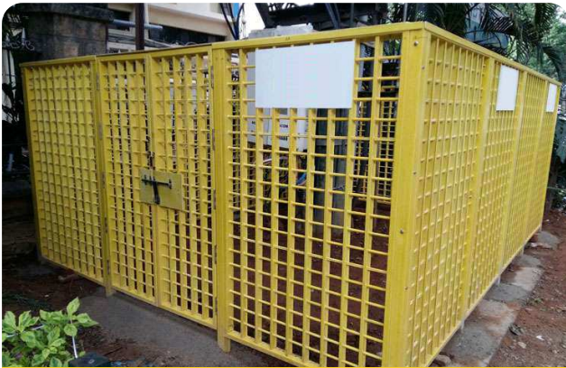
Electrical Substation Guardrail
