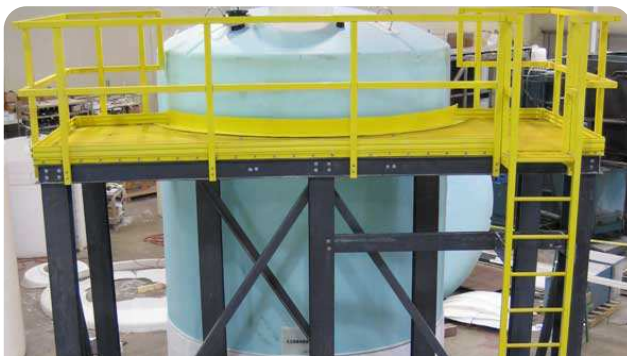
FRP fixed ladders for platform access
