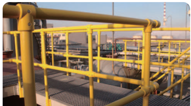
Round Handrails Platform
